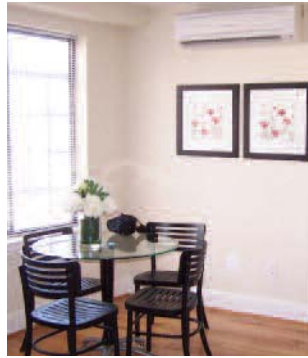
Split system air handler located in living area.
