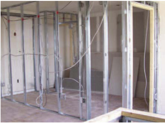
Above: AireShare™ ventilators were used in metal stud walls which separate bedrooms from living areas.
