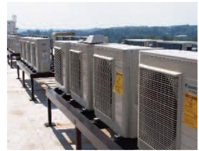
Split system condensers installed on roof.
