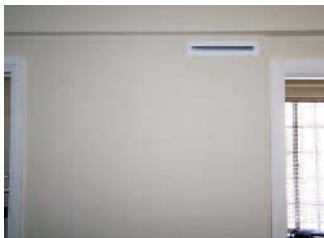
Above: Low profile diffuser is located near ceiling in the bedroom.
