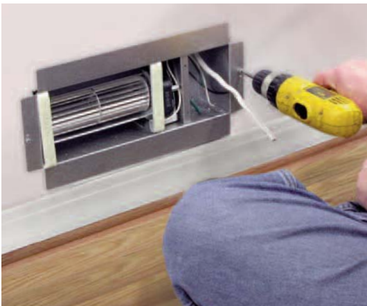
Below: AireShare™ fan is being installed in cutout between wall studs and hardwired.
